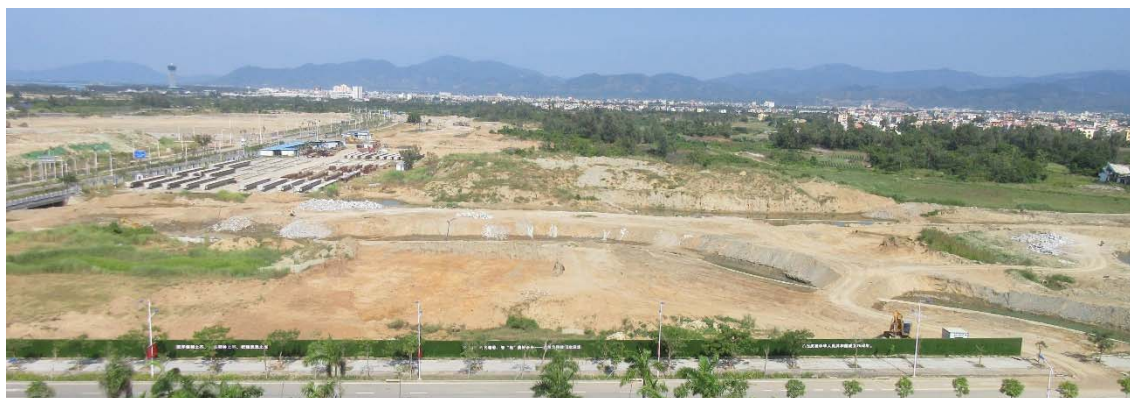
Figure 1. A construction site for a new marine industrial city in the suburbs of Sanya City, Hainan Province. Taken from the 9 th floor of the incubation building with sea on the left. University Campuses such as Shanghai Jiao Tong University are on the other side of the forest on the left. Construction work on Shanghai Jiao Tong University is scheduled for 2020.
